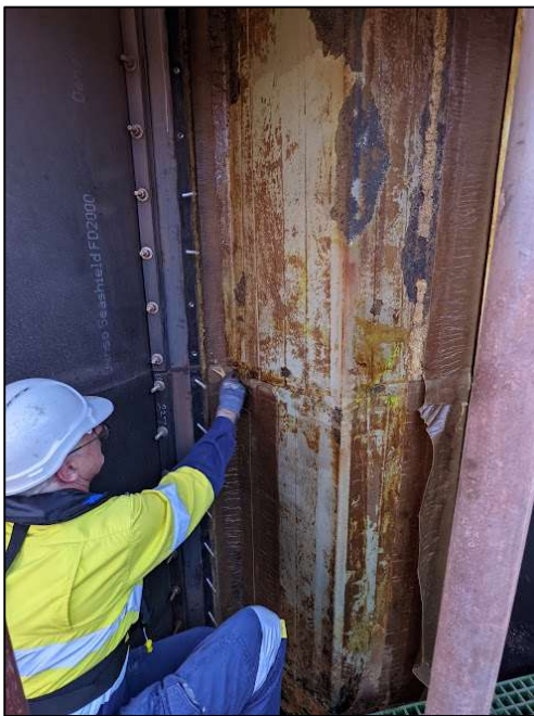
Figure 4. (1) Inspection of a trial after 2 years; (2) the outer covering, foam blocks and petrolatum tape have been removed for inspection of the steel surface; and (3) the petrolatum primer is still in place on the steel surface and water ingress has not occurred.
